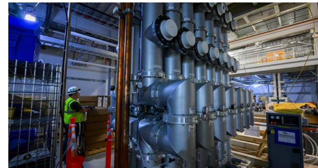
Figure 5: RF coax installed at the SPARC facility for transmitting the RF power from the plant to the plasma
