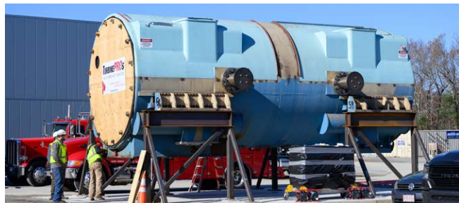
Figure 4: Stator from the Constellation Energy Mystic Generating Station on a temporary storage stand at the SPARC site. The stator will soon be installed in the energy storage building along with the rotor and flywheels.
