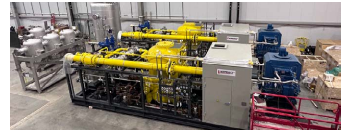
Figure 6: Cryoplant main compressors and oil removal system installation in the SPARC Utility Building.
