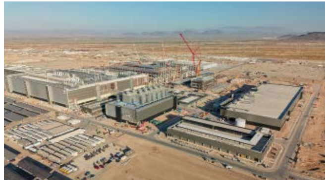
Fig. 8. TSMC facility under construction in Phoenix, Arizona (TrickHunter, CC BY-SA 4.0, via Wikimedia Commons).
